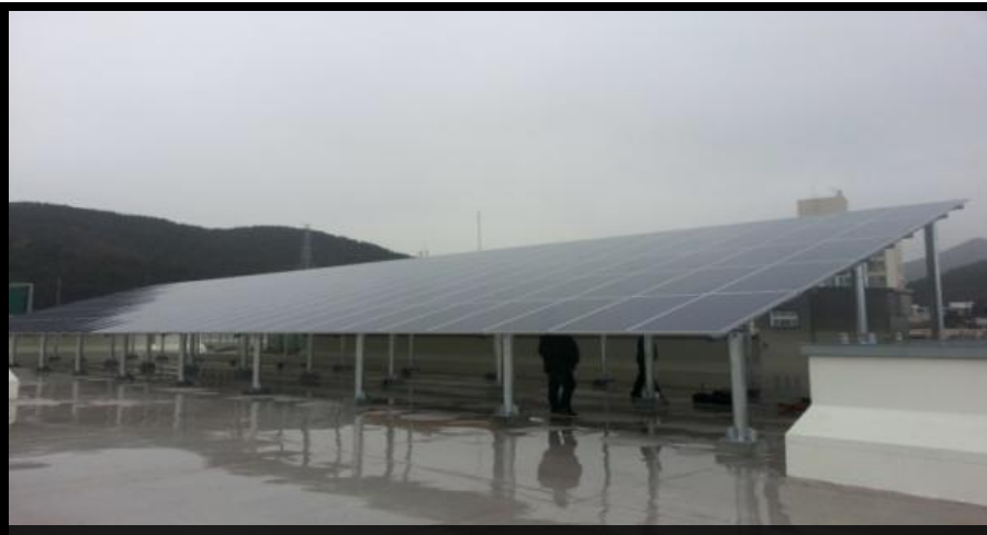
Busan Elementary School 71.5 kW
