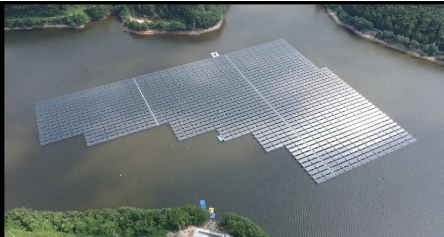
2.0MW Floating Solar Power Plant at Mabuk Reservoir in Pohang
